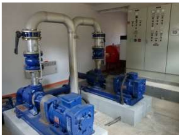
Figure 10 : Station de reprise (Source : SMDE)
